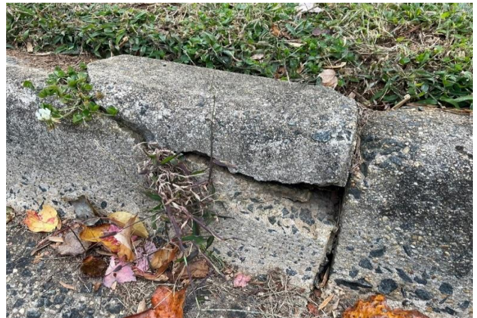
Damaged concrete curb
