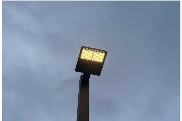
Light fixture atop pole
