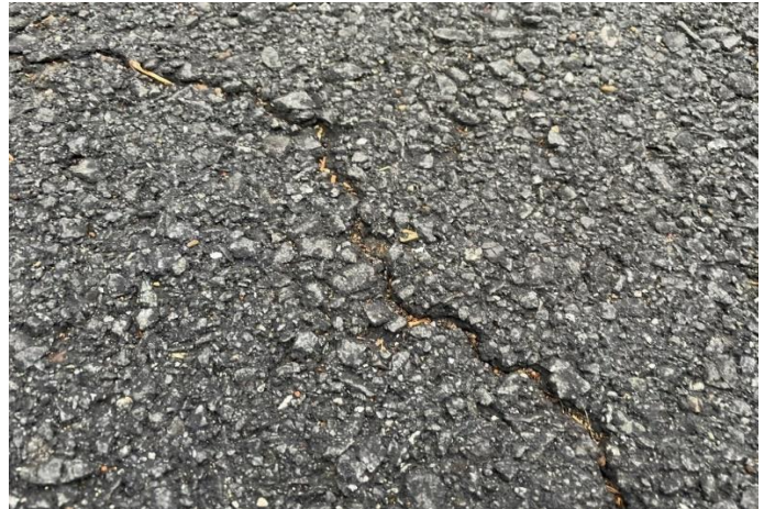
Crack at asphalt
