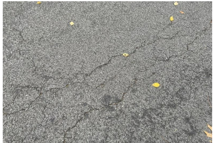
Cracks at asphalt pavement
