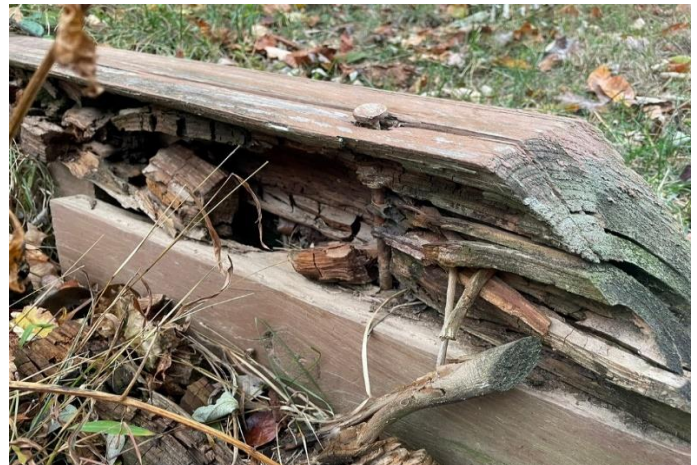
Rotten and damaged timber
