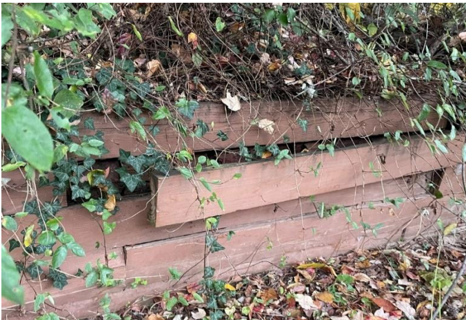
Damaged timber at retaining wall
