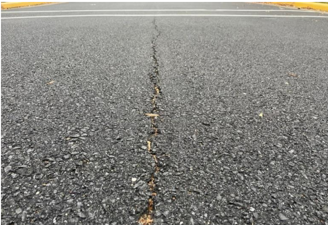
Crack at asphalt pavement
