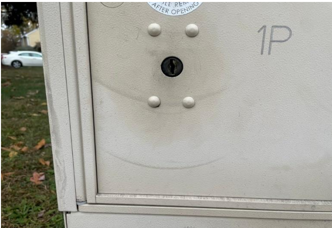
Minor surface damage at parcel box
