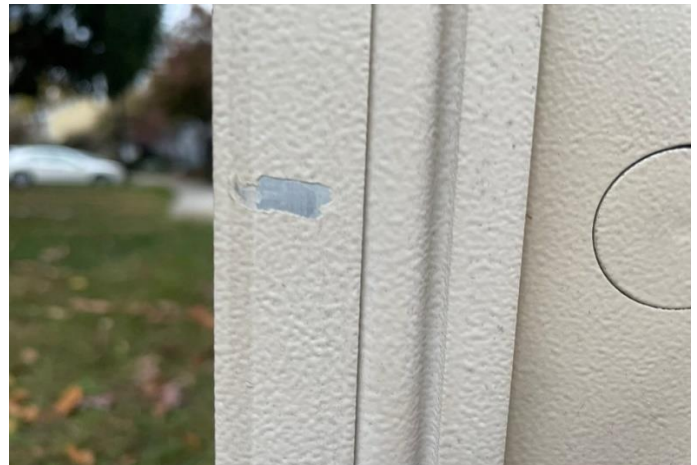
Minor surface damage
