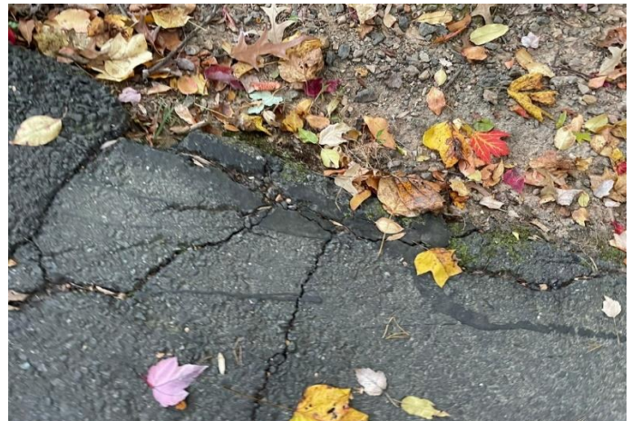
Cracks at asphalt path
