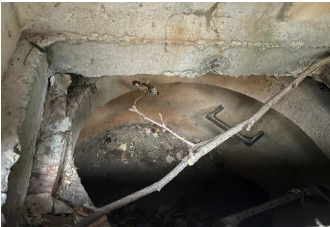
Debris at catch basin interior
