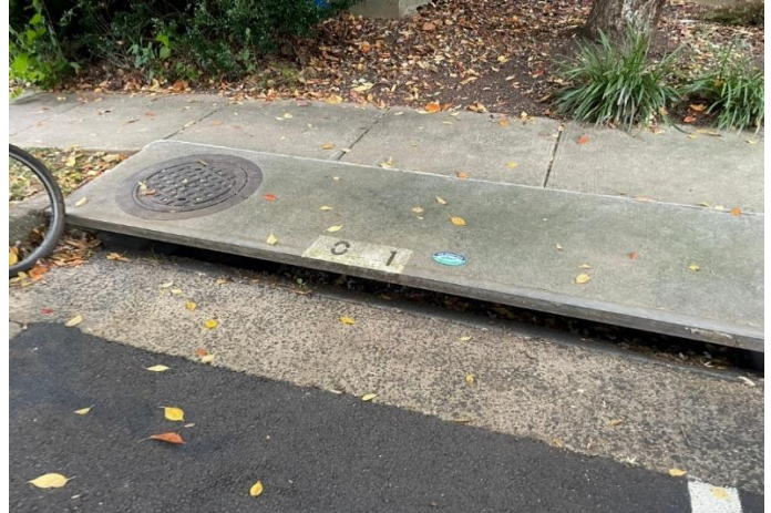
Typical catch basin
