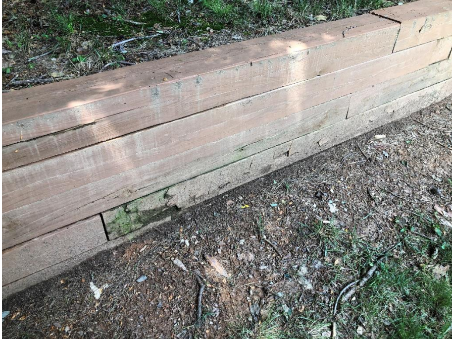
Photograph 11 – Deteriorated timber along base of retaining wall
