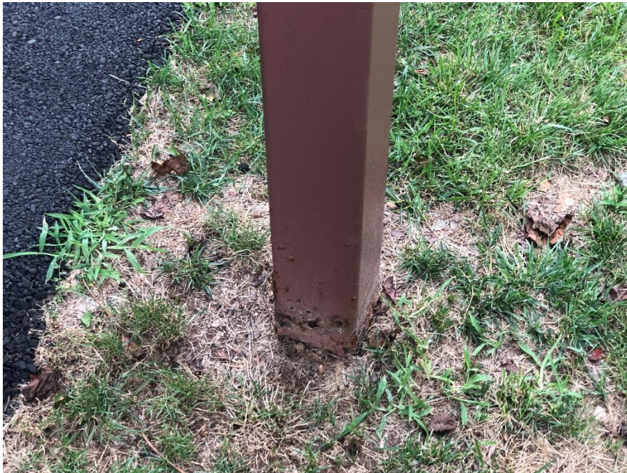
Photograph 14 – Corrosion at base of light post
