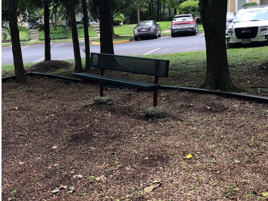
Photograph 9 – Exposed bench concret footings presenting safety hazard
