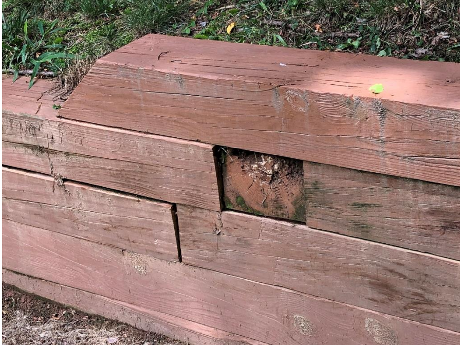
Photograph 13 – Deteriorated end of retaining wall tie-back timber
