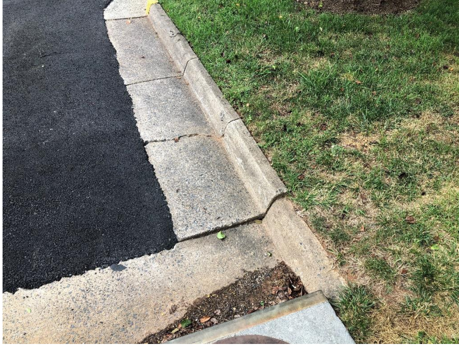
Photograph 5 – Cracked section of curb and gutter assembly
