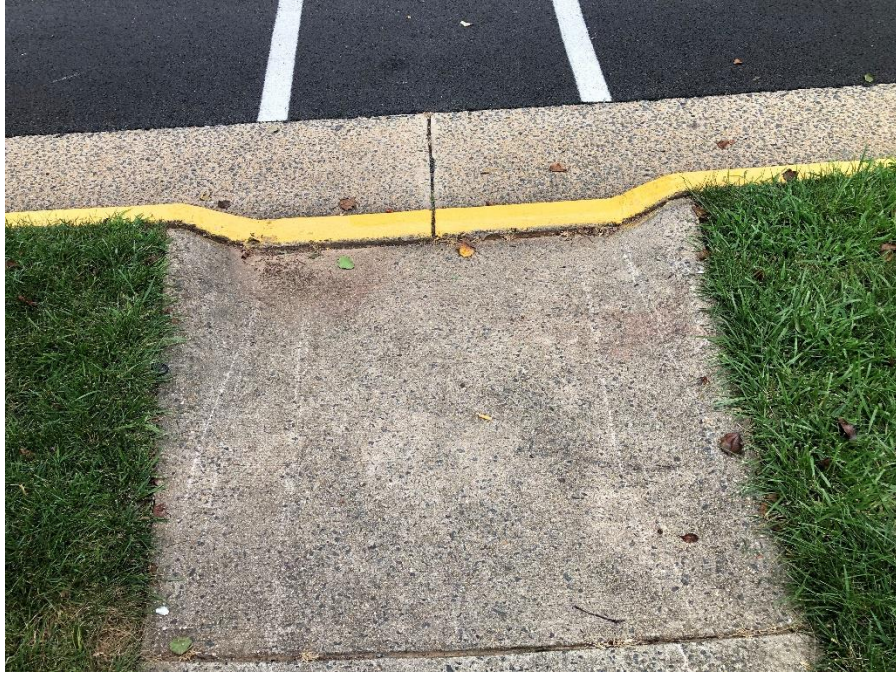
Photograph 3 – Sunken section of sidewalk
