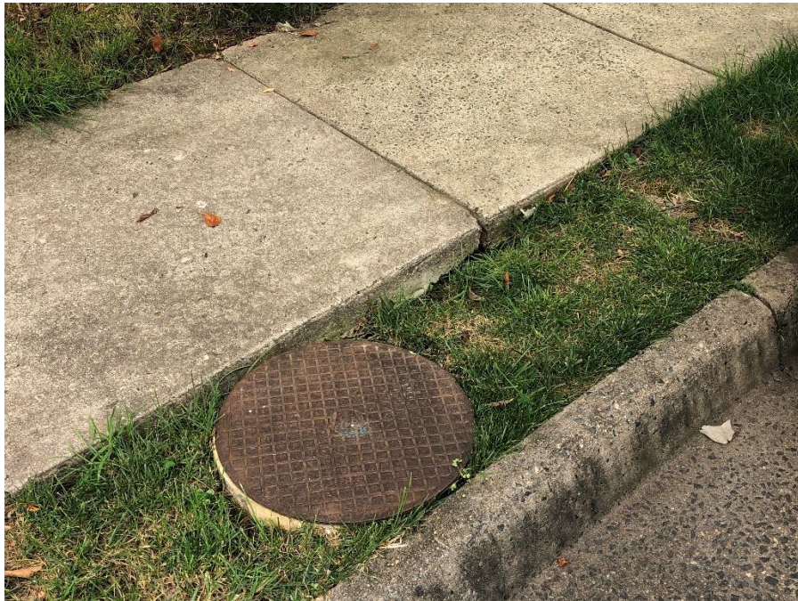
Photograph 4 – Sunken ground between sidewalk and curb – note sidewalk undermined
