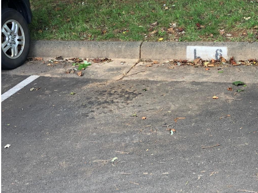
Photograph 1 – Stainng on pavement from automotive fluid
