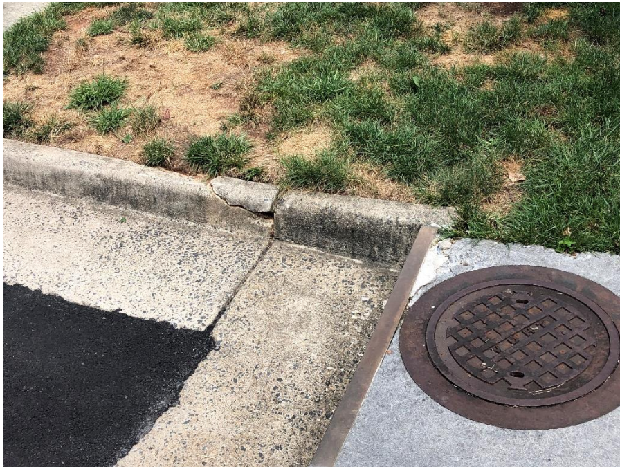
Photograph 6 – Broken section of curb and gutter assembly
