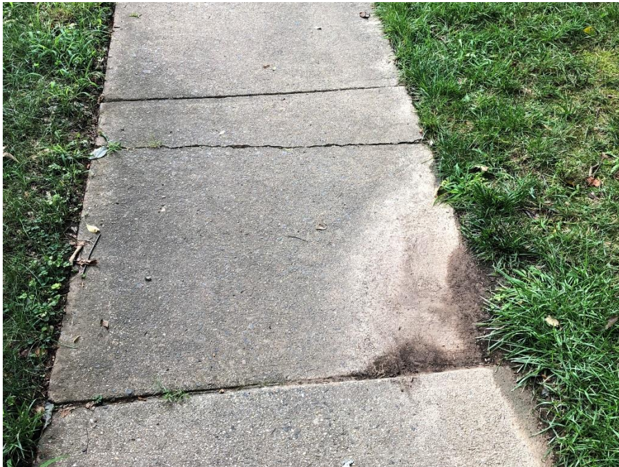
Photograph 2 – Crack in sidewalk
