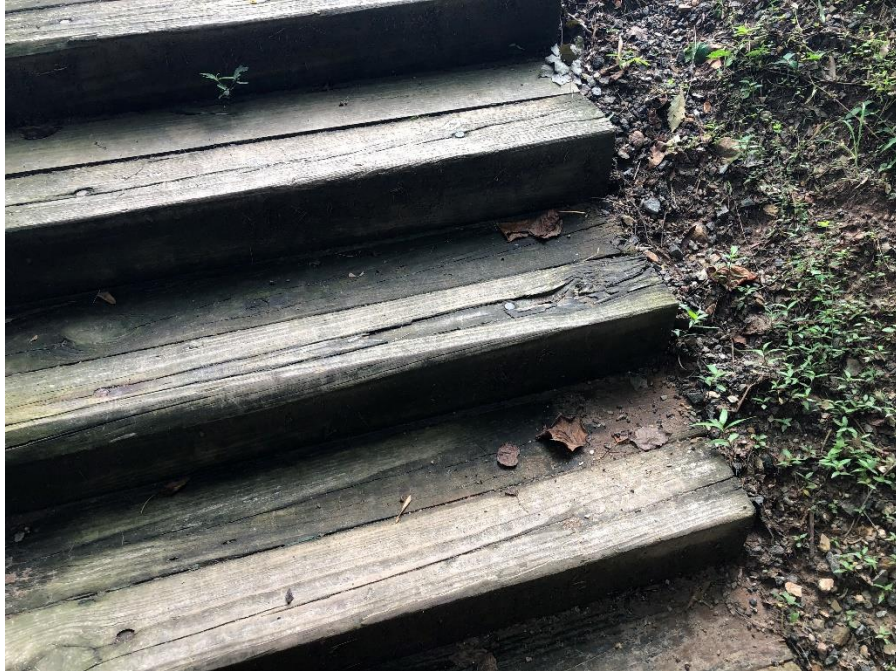
Photograph 7 – Deteriorated timber in stair assembly
