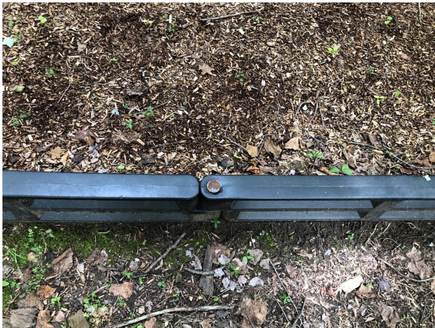
Photograph 10 – Corrosion on tot-lot border spike
