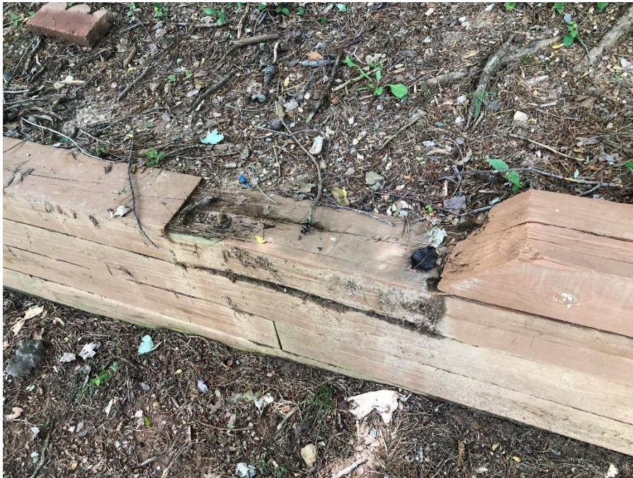
Photograph 12 – Deteriorated timber along top of retaining wall
