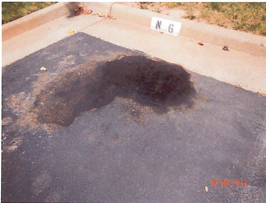
Photograph 2 – Automotive fluid on asphalt pavement.
