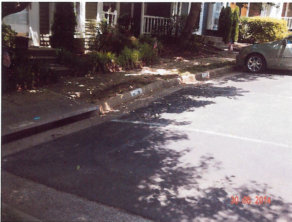
Photograph 6 – Sunken pavement and curb and gutter at storm water inlet.
