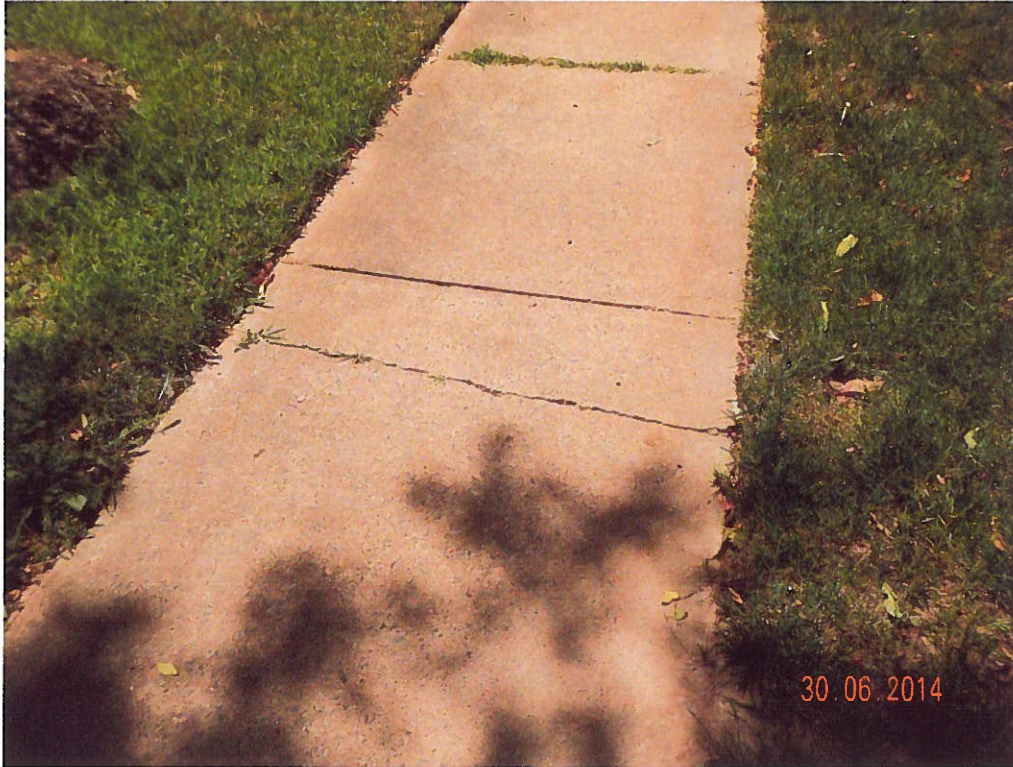
Photograph 3 - Crack in concrete sidewalk.
