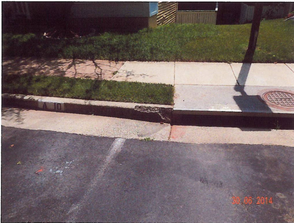
Photograph 5 – Broken curb and gutter assembly.
