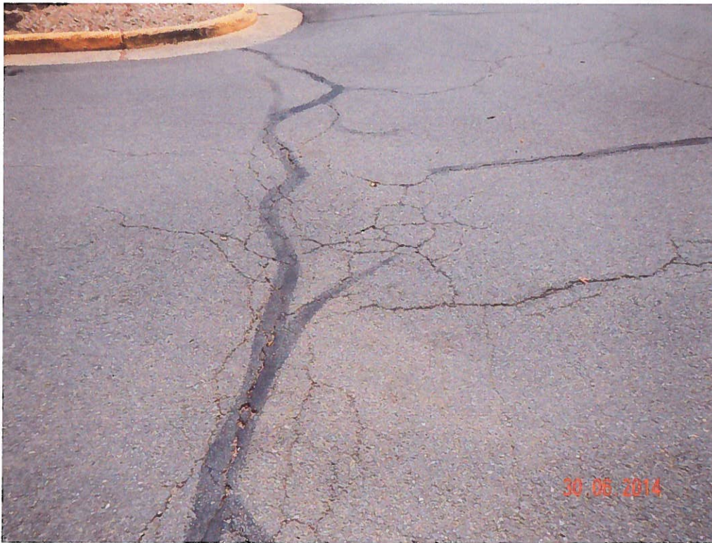
Photograph 1 – Interconnected cracking in asphalt pavement.
