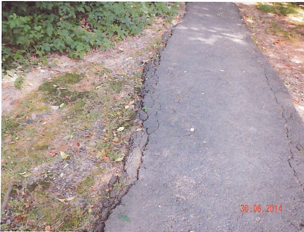
Photograph 8 – Cracked, broken asphalt foot path.
