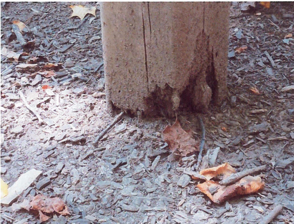
Photograph 10 – Decayed equipment support timber at tot-lot.
