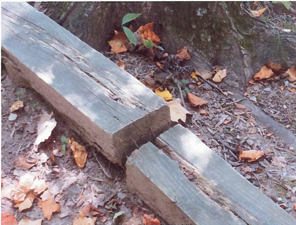
Photograph 12 – Uplifted landscaping timber at tot-lot.
