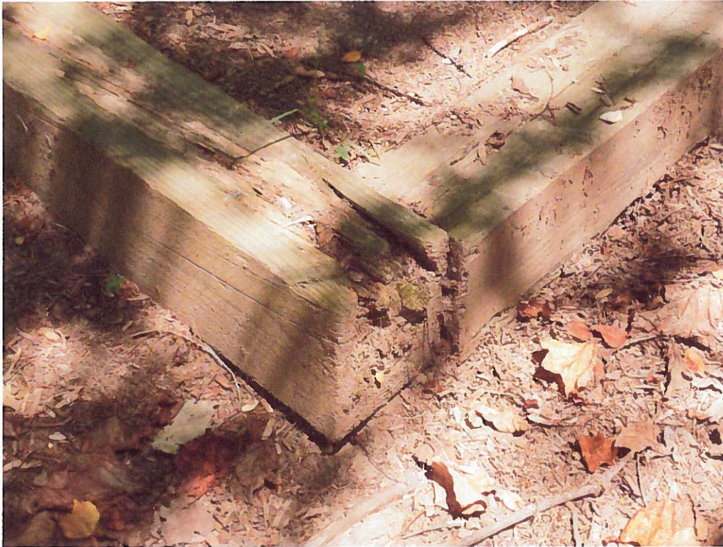
Photograph 11 – Decayed landscaping timber at tot-lot.
