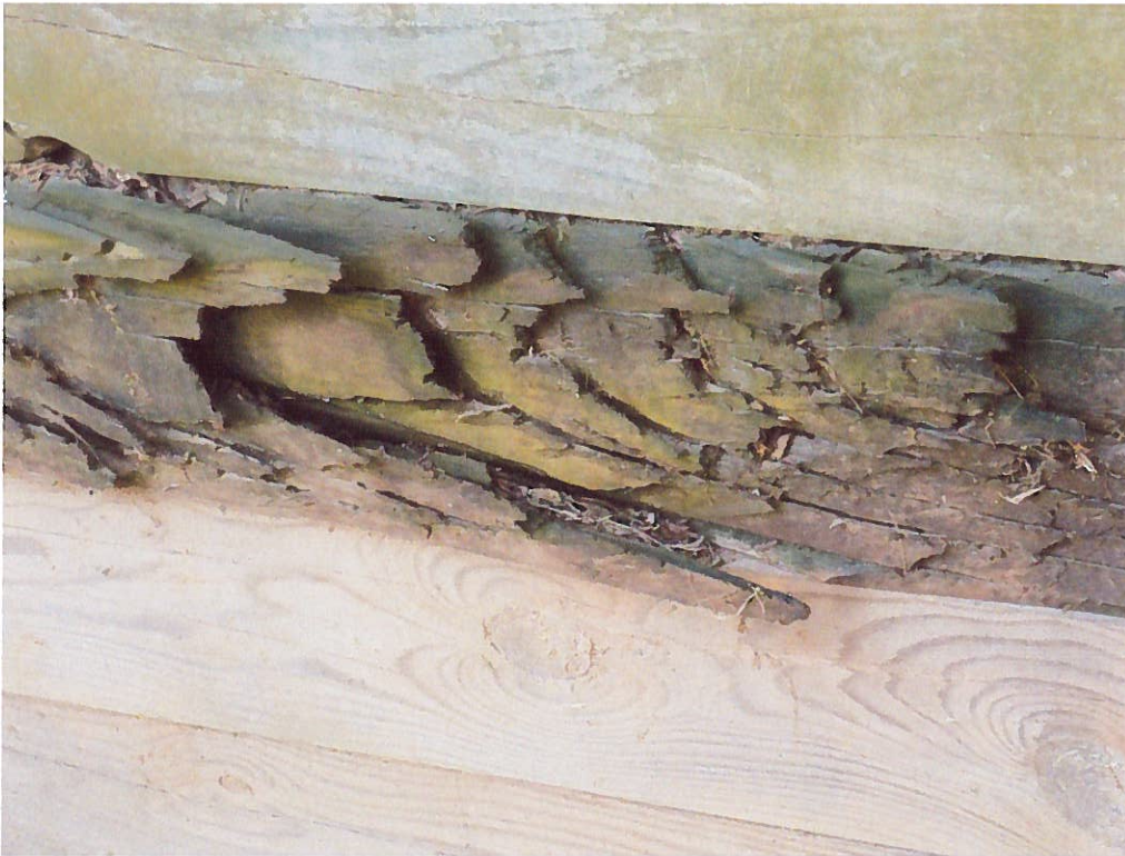
Photograph 13 – Severely checked/splintered retaining wall timber.
