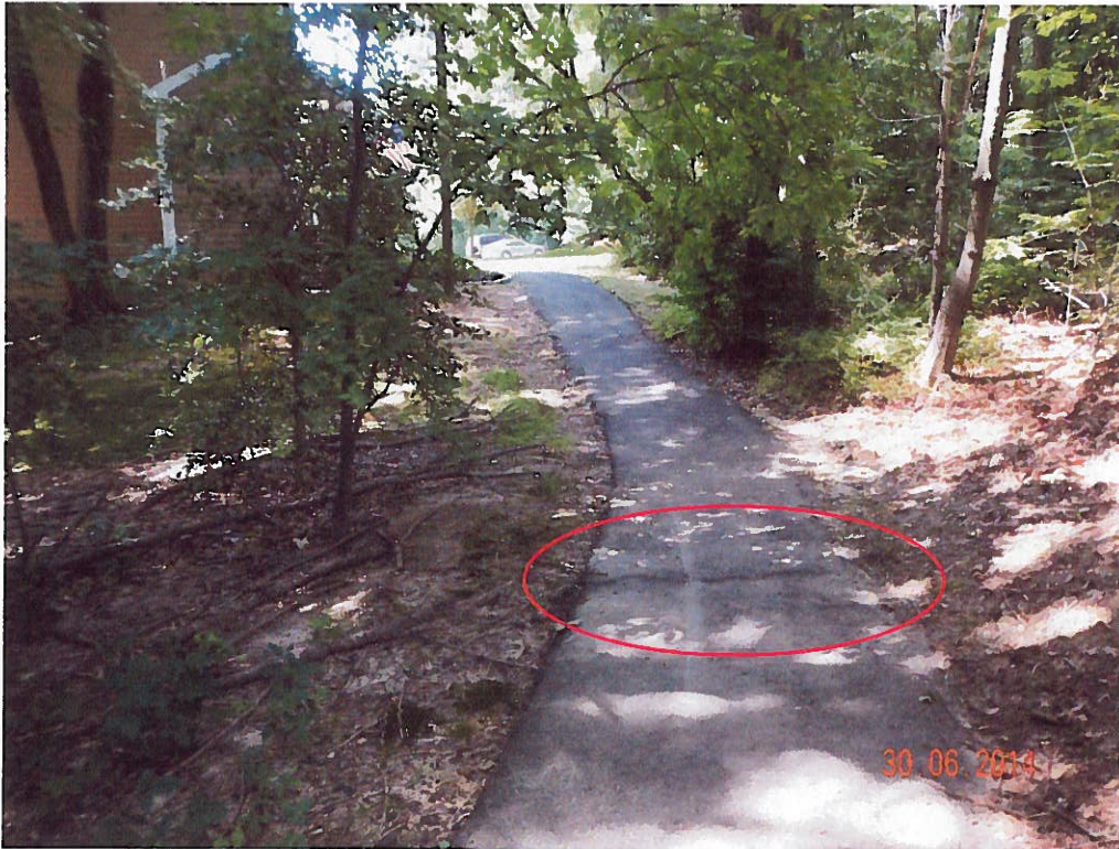
Photograph 7 – Asphalt foot path uplifted by tree root.
