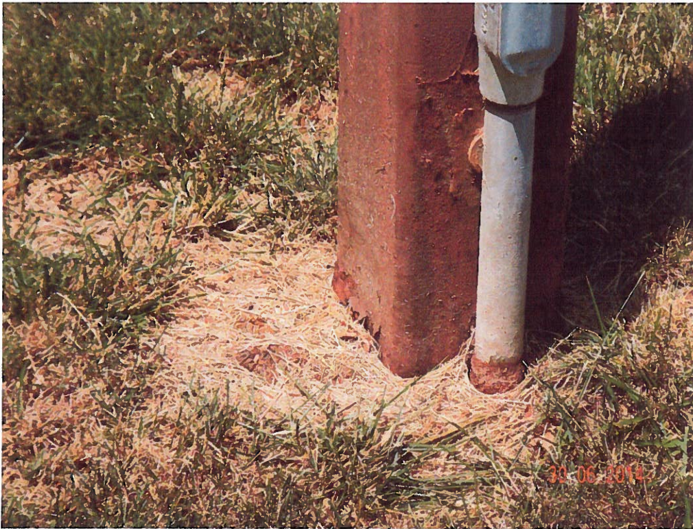
Photograph 14 – Typical rusted light post and electrical conduit.
