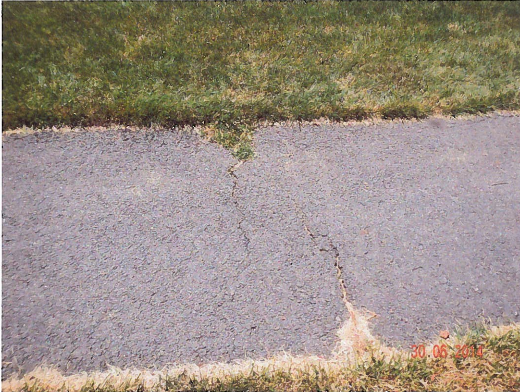
Photograph 9 – Plants in cracked asphalt foot path.
