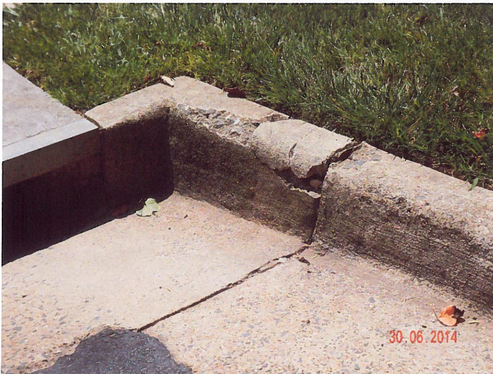
Photograph 4 - Broken curb and gutter assembly.
